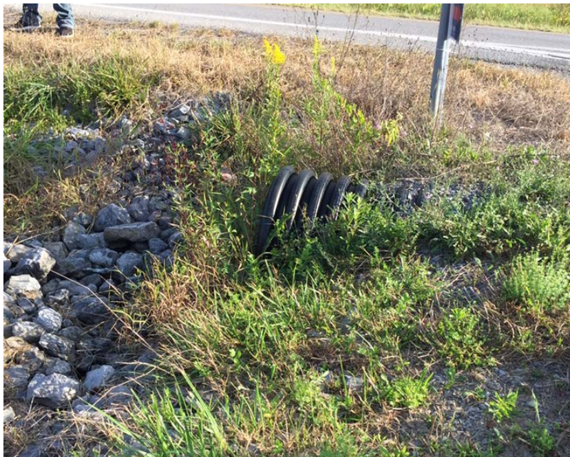
Figure 8: Culvert at the Intersection of Station and Fairgrounds Road Photo by Michael Henderson
